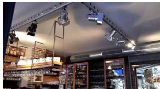
Trattoria Restaurant U-Match; Duct France
